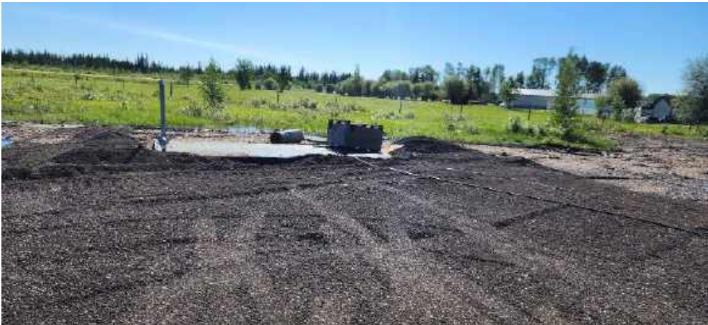
This is the cistern area to be covered by the Accessory Building.
